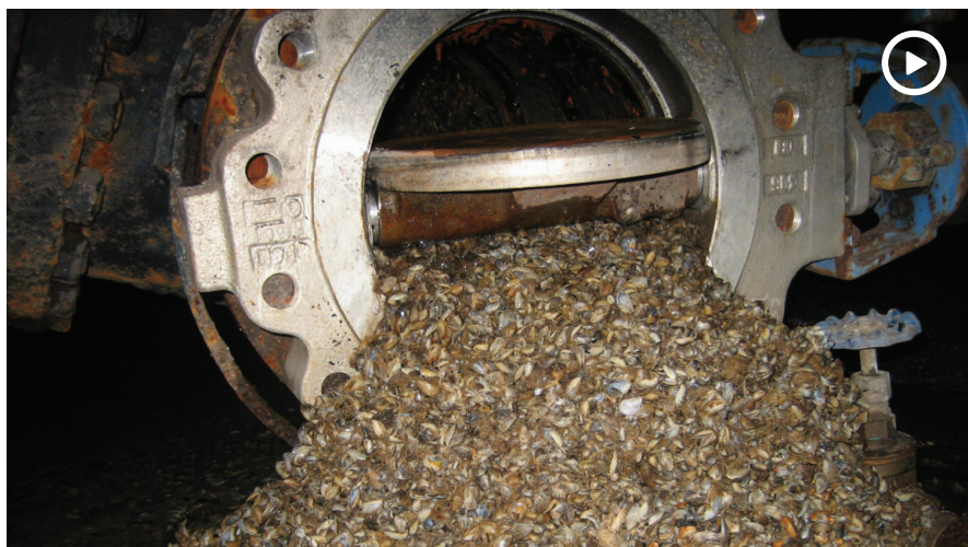
Mussels have infested the penstock belly drain at a Lower Colorado River dam (see video at HydroWorld.com ).
